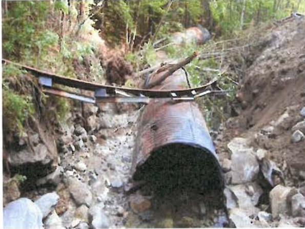
Road failure at a 3-m culvert placed within a 6-m bankfull width stream, GMNF
