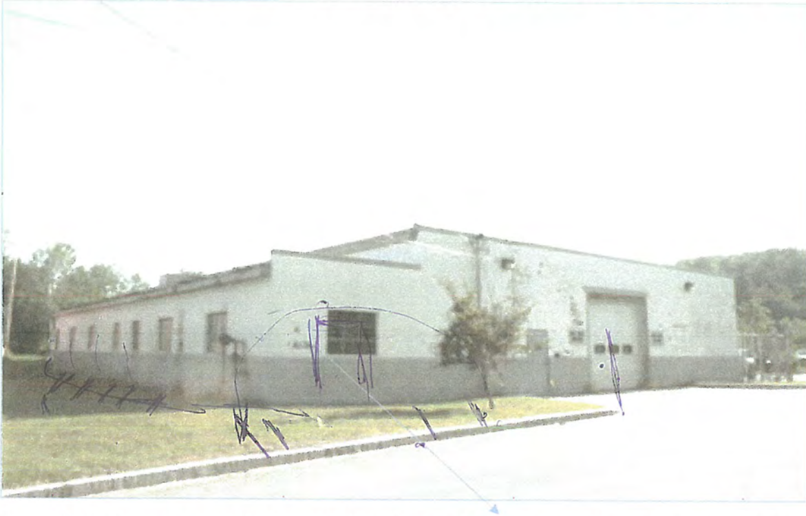
New office entrance door to replace existing window. Engineering and Architecture being done by SK Engineering. Overhead Garage door to be framed in with new double doors. Front parking configuration being done by SK Engineers
