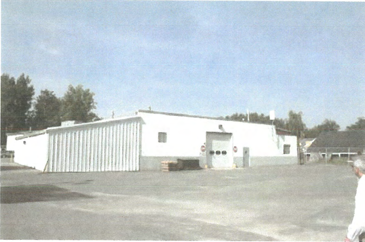
Rear of building. Overhead garage door to be framed in with double doors.
