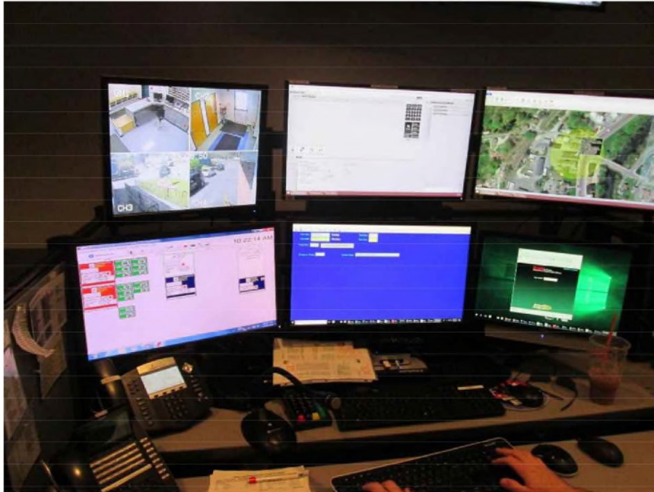
Figure 7.4: Data Systems and Controls Available at Dispatch Position.
